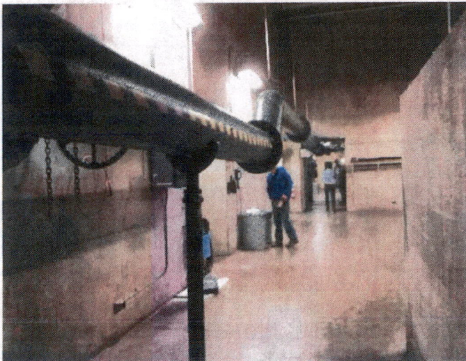
Figure 2.4 12-inch Pipeline from Penstock to Raw Water Pump
