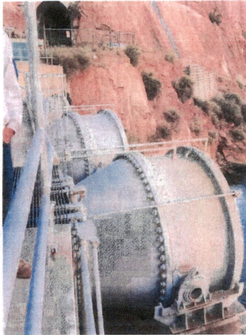
Figure 2.11 Hollow Jet Valves and Entrance to the Access Tunnel
